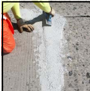
The polymer slurry can now be feathered into the existing concrete ensuring a smooth ride with no bump.
