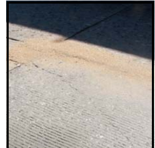
Once fully cured, the area can then be returned to traffic, sometimes in less than 30 minutes
