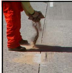
Broadcast the supplied 12 pounds of topping sand over the area to create a high traction surface.
